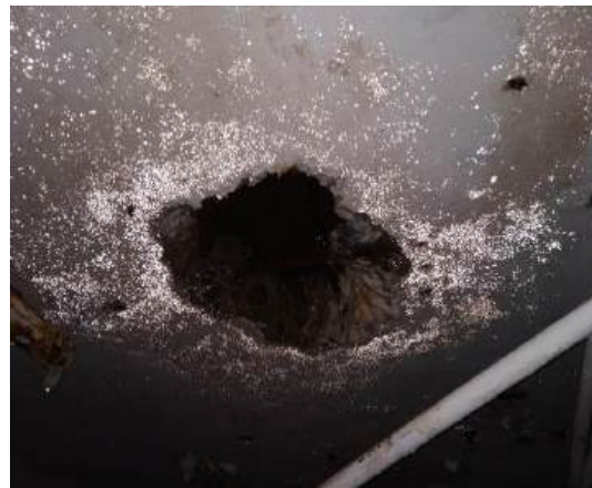
(d) Hole in ceiling outside of Store room(9)
