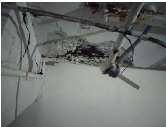
(c) Spalled concrete with R/f exposure and loose cover in beam at next to store room(9) and light control
