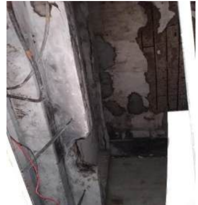
(b) Presence of loose cover & a part of concrete is missing.
