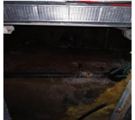
(j) Presence of moisture, blisters and leakage on beam in recording room(17)
