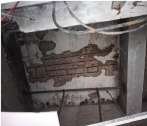
(a) Spalled concrete with exposed R/f in slab at ladies toilet of Dariya Sangam
