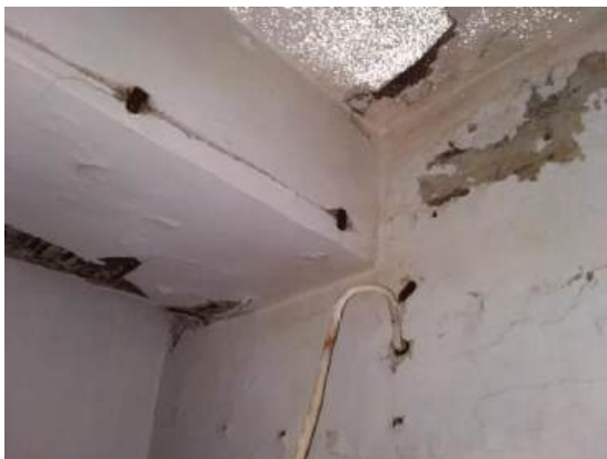
(g) Delamination in beam located in room(9)
