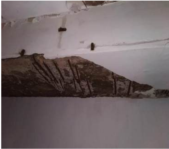
(f) Delamination at store room(9)(f) (f) Delamination of slab at store room(9)
