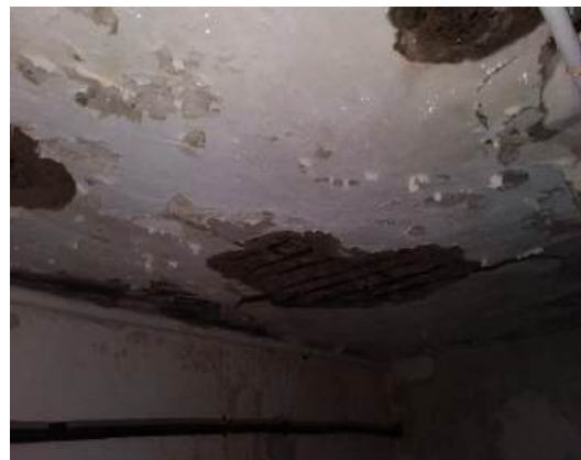
(h) Spalled concrete with exposed R/F in room (9)
