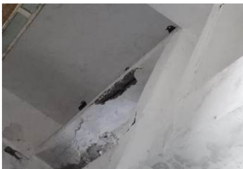
(c) Spalled concrete with R/f exposed in the ventilation projection of Generator room(81)
