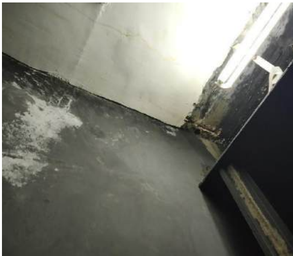
(a) Spalled concrete with R/f exposed in slab at the entrance of black box
